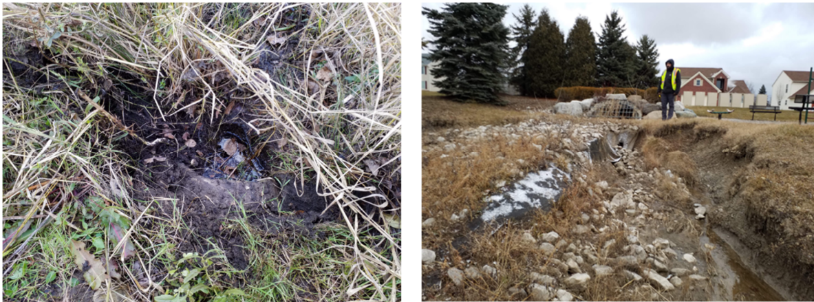
Figure 2-6 Sediment and Erosion issues (Left) Excessive sediment deposition at basin inlet BV-03S08E27NENW-1. (Right) Basin RM-03S09E09NWNE-1 has devastating shoreline erosion near its largest inlet, and the water from this inlet has eroded away the basin's spillway (not pictured).
