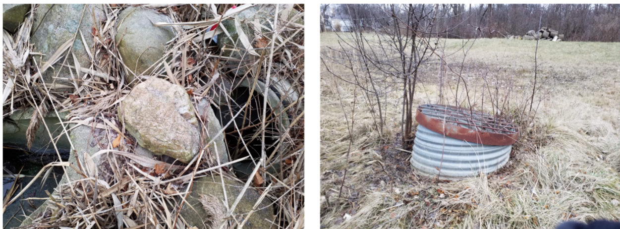
Figure 2-4 Detention Basin Maintenance Examples (Left) detached inlet end section from basin TY-03S10E27SWNW-2, (right) crooked standpipe from basin SG-03S10E35SWNW-1.
