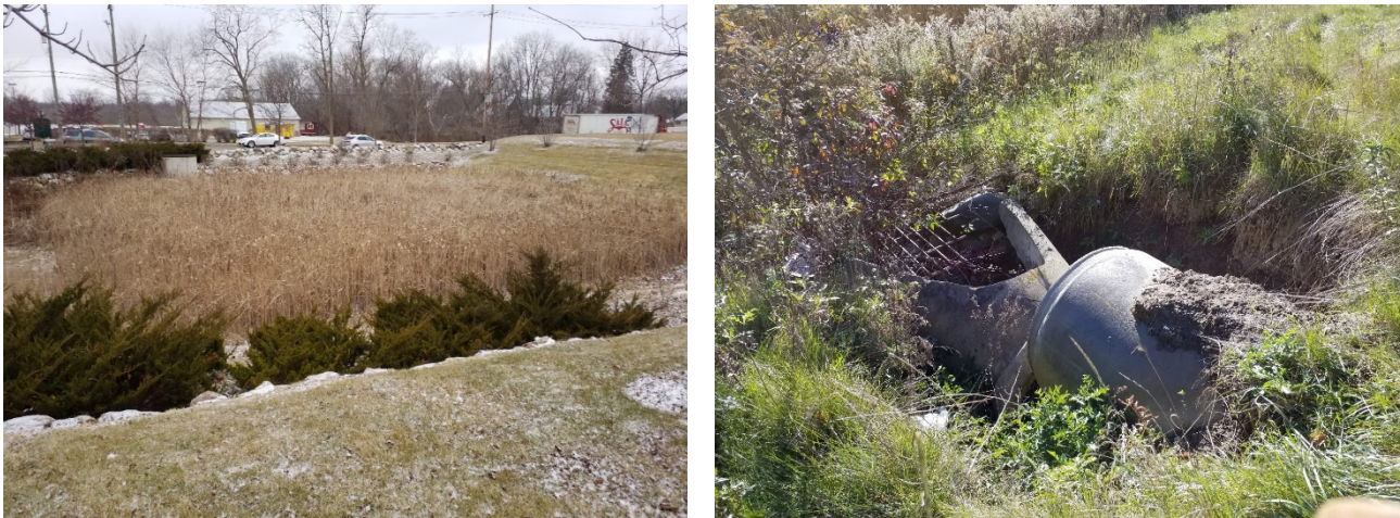
Figure 2-7. (Left) Detention Basin with invasive vegetation; (Right) Dislodged end section with severe erosion
